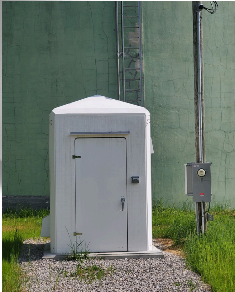
Pictured Above: Control Building for the Debord Hill Tank Mixer. All tank mixer components are contained within the tank in the background.
