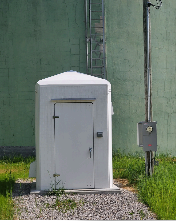
Pictured Above: Control Building for the Debord Hill Tank Mixer. All tank mixer components are contained within the tank in the background.
