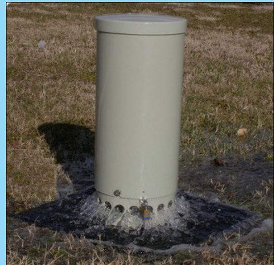
Pictured Above: Auto flushing device in operation.
